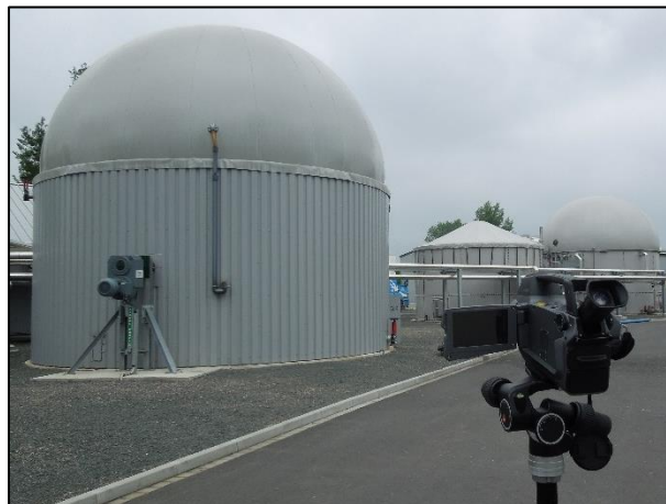
Figure 1: Leakage identification with IR-camera at a biogas plant (© Torsten Reinelt, DBFZ)
