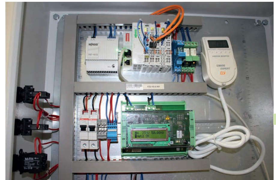
Fig. 12 Wind turbine electrical cabinet with grid monitoring and provision of measurement data to the gateway
