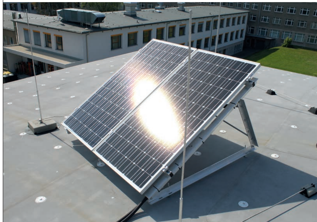
Fig. 10 Photovoltaic plant in the DBFZ test field
