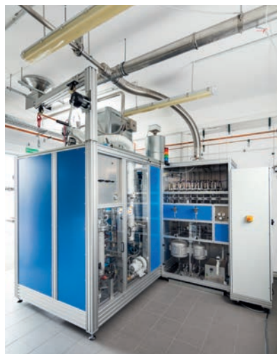
Fig. 51 Fixed-bed gasifier at the DBFZ's fuel technical centre
