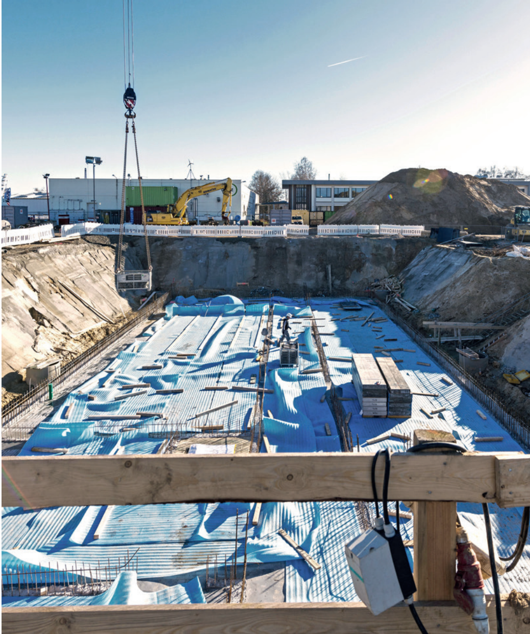
Fig. 57 Excavation pit for the new office building and event centre on the DBFZ site (Autumn 2016)
