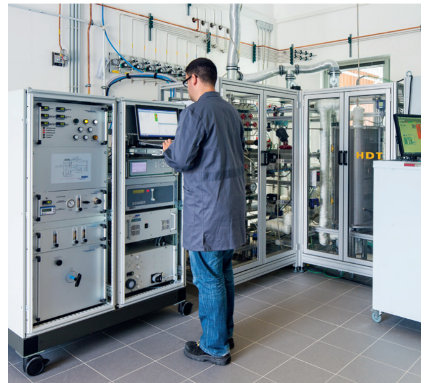
Fig. 36 Work in the DBFZ fuel technical centre
