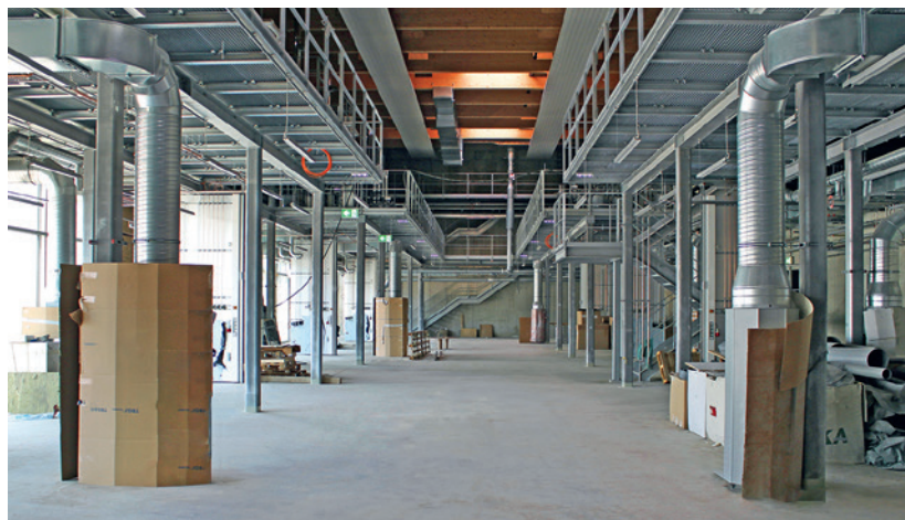
Fig. 43 New technical centre of the DBFZ (thermo-chemical conversion part) in April 2019
