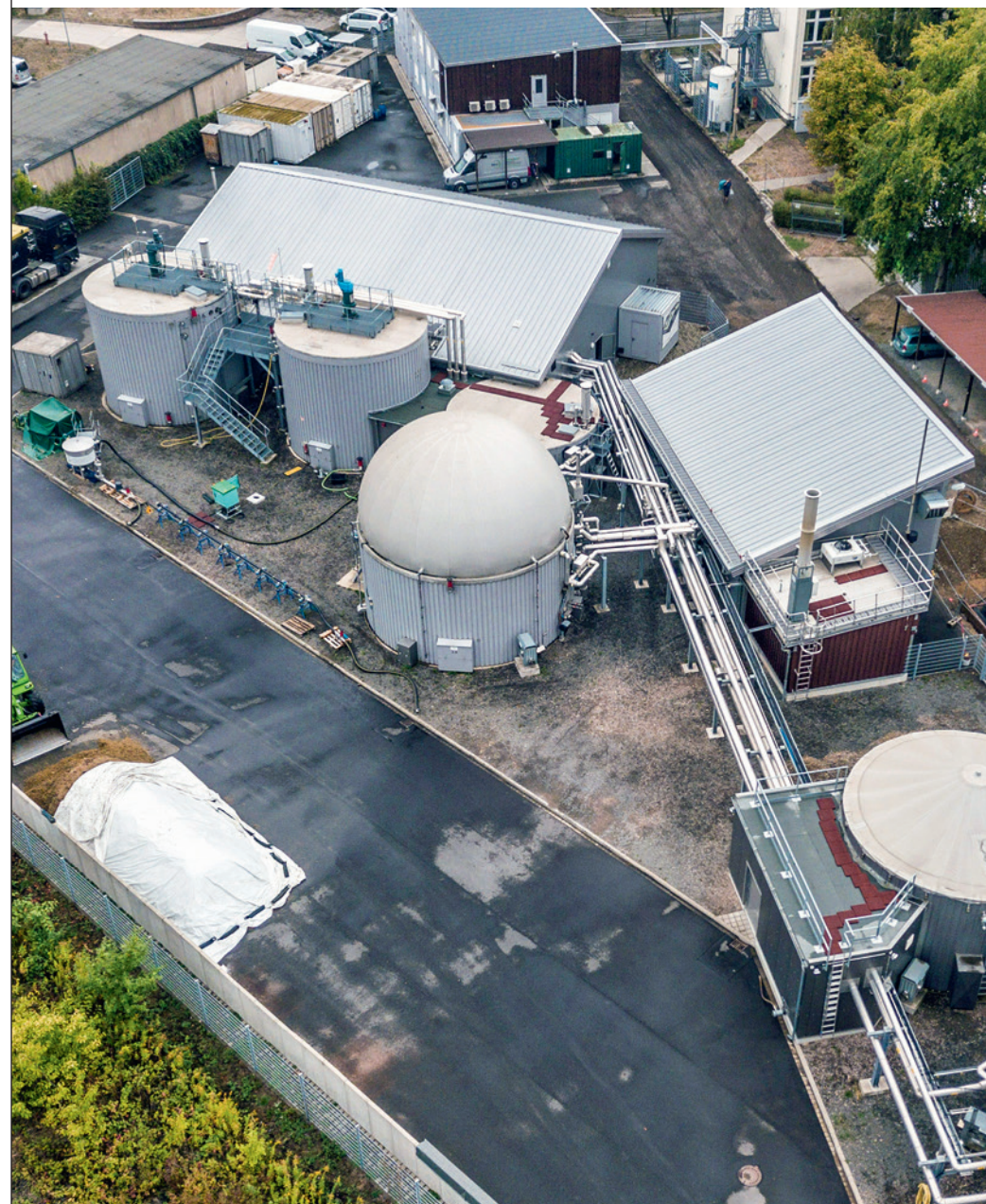
Fig. 42 The DBFZ research biogas plant
