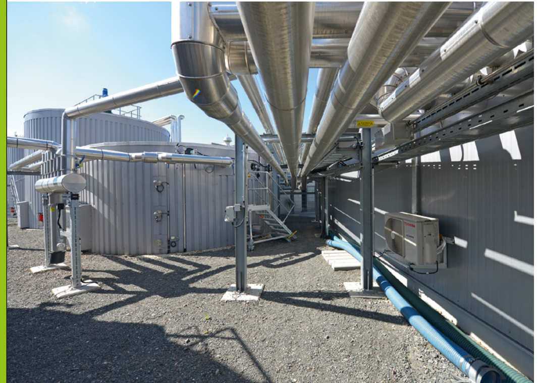
Fig. 40 The research biogas plant
