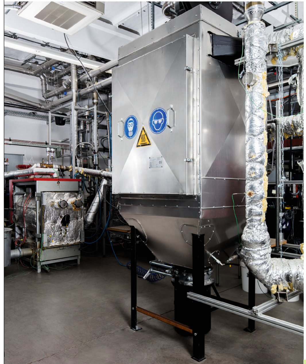
Fig. 37 Multifuel boiler in the combustion lab of the DBFZ
